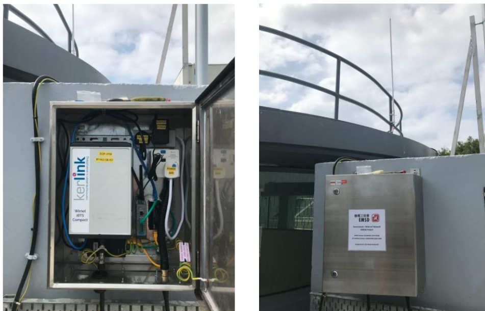
Figure 5. On-site deployment of LoRa gateway
